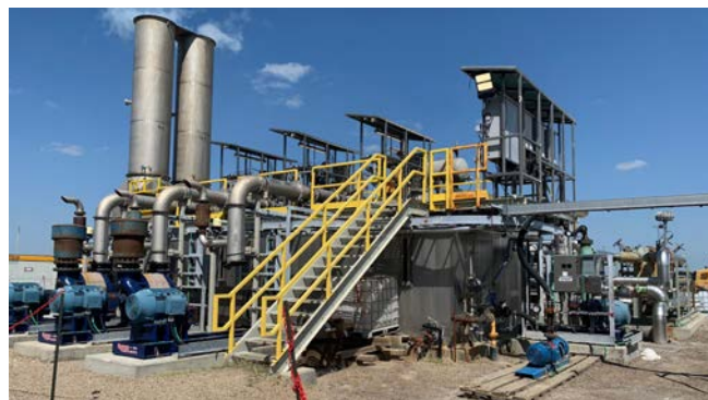
Heating exchange setup at the Milestone Project
