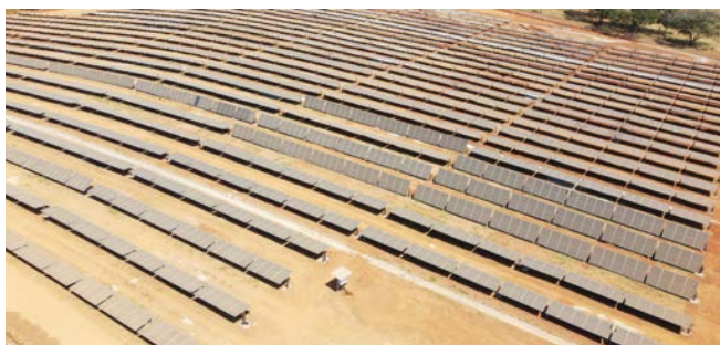
Omnigen solar panels
