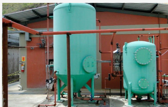
Water treatment plant at Atlantic Nickel
